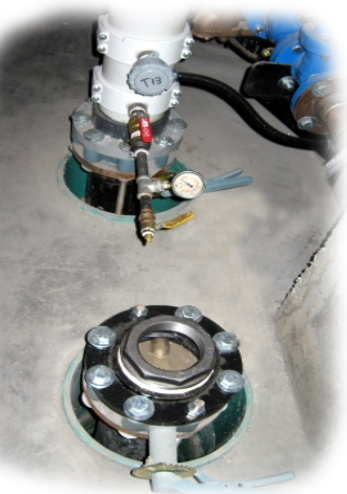
Geo-thermal supply and return lines
